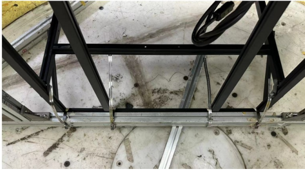
Panel cable ties fixed
